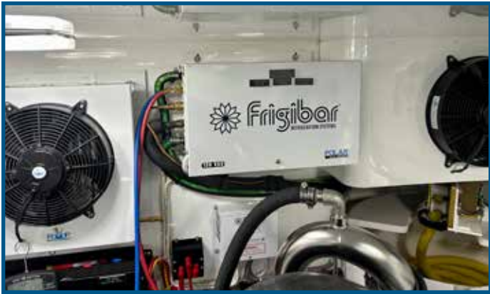
Below: Frigibar components support refrigerated and freezer systems throughout the boat.
