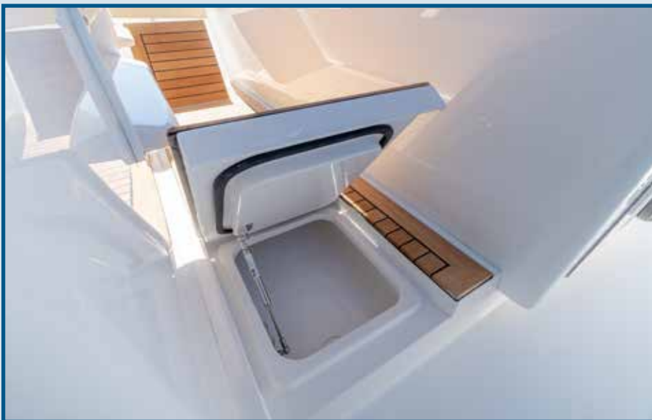
A variety of areas on a V-46 that utilize systems from Finish Mechanical at Viking Mullica: climate-controlled cabin, refrigerated mezzanine box and helm platform drink box.
